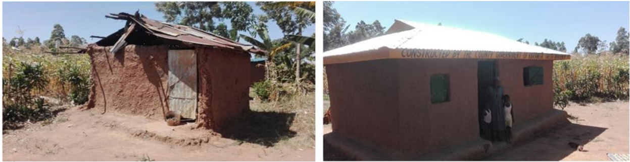
Photo 1: A county resident's house before and after county intervention
