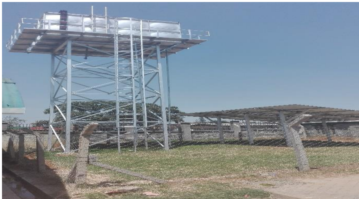
Photo 8: Butere Market water supply project with a solar pumping unit
